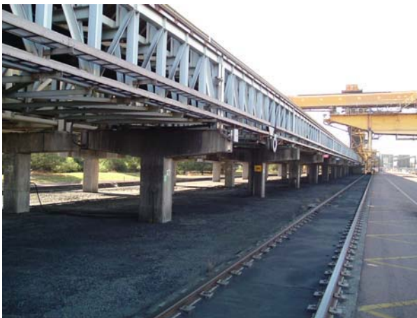
Figure 1. Typical Large Conveyor Belt System.
