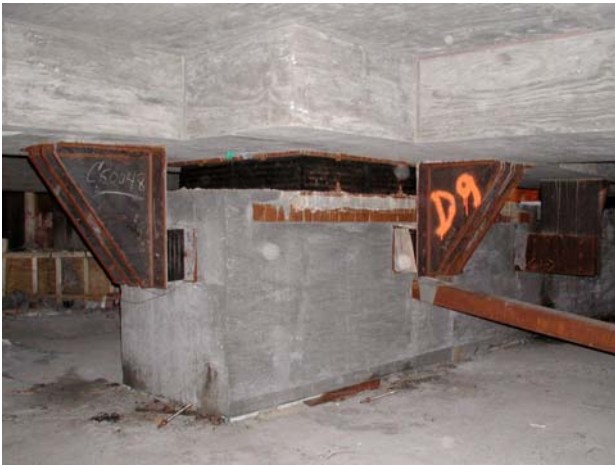
Figure 5 Jazz@Lincoln Center photo showing concrete encased steel beams and isolation bearing pads
