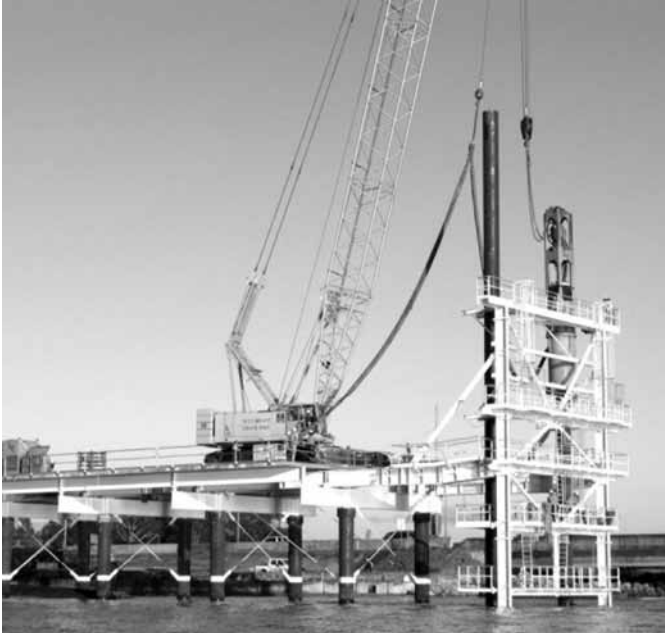
Figure 1: Photo of a temporary pile being driven at Pier 2. The existing Houghton Highway bridge can be seen in the background.
