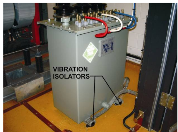
Figure 6. Isolating Transformer with vibration isolators installed
