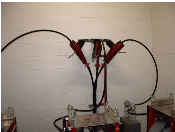
Figure 3. LCFI cell power cables mounted on FIR wall
