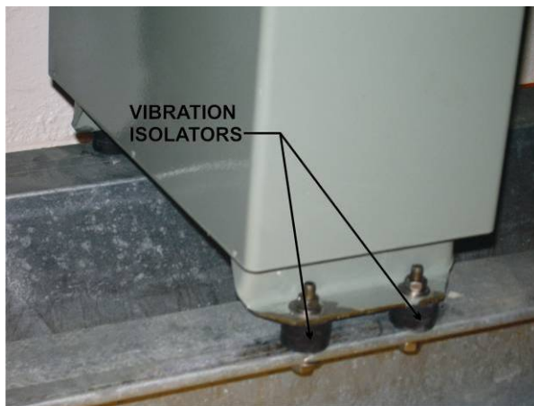
Figure 8. Capacitors with vibration isolators installed
