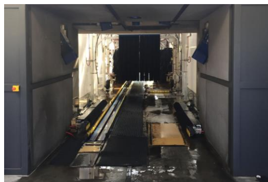
Figure 2: Exit from the car wash, with drying section at the front and wet section at the back
