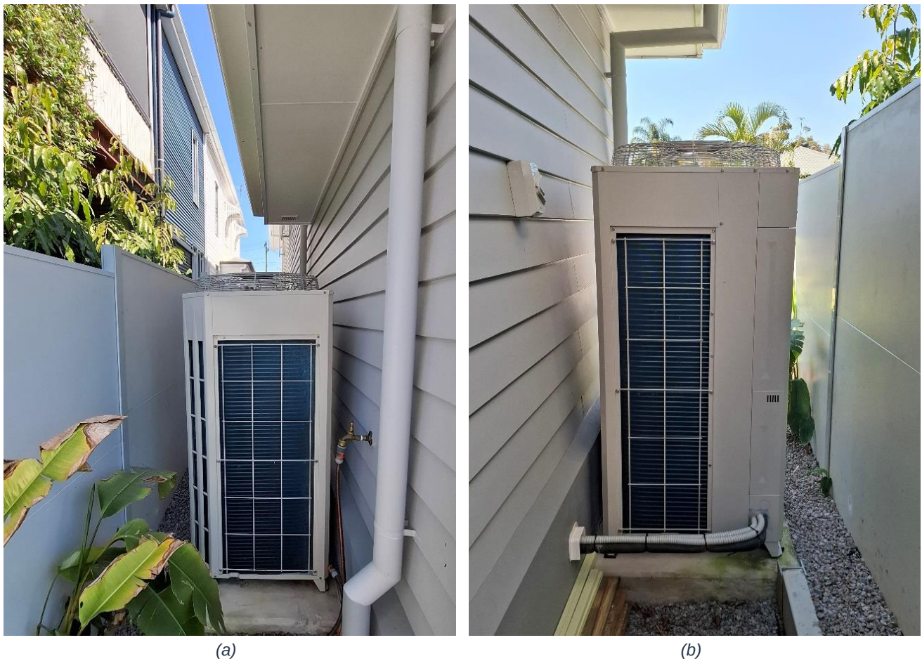
Figure 2 – A typical problematic residential air-conditioner installation
