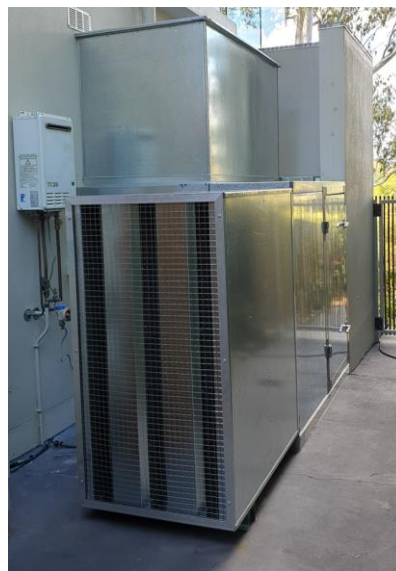
(b) 18 kW condenser with enclosure
