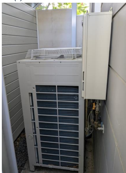
(c) 25 kW condenser untreated
