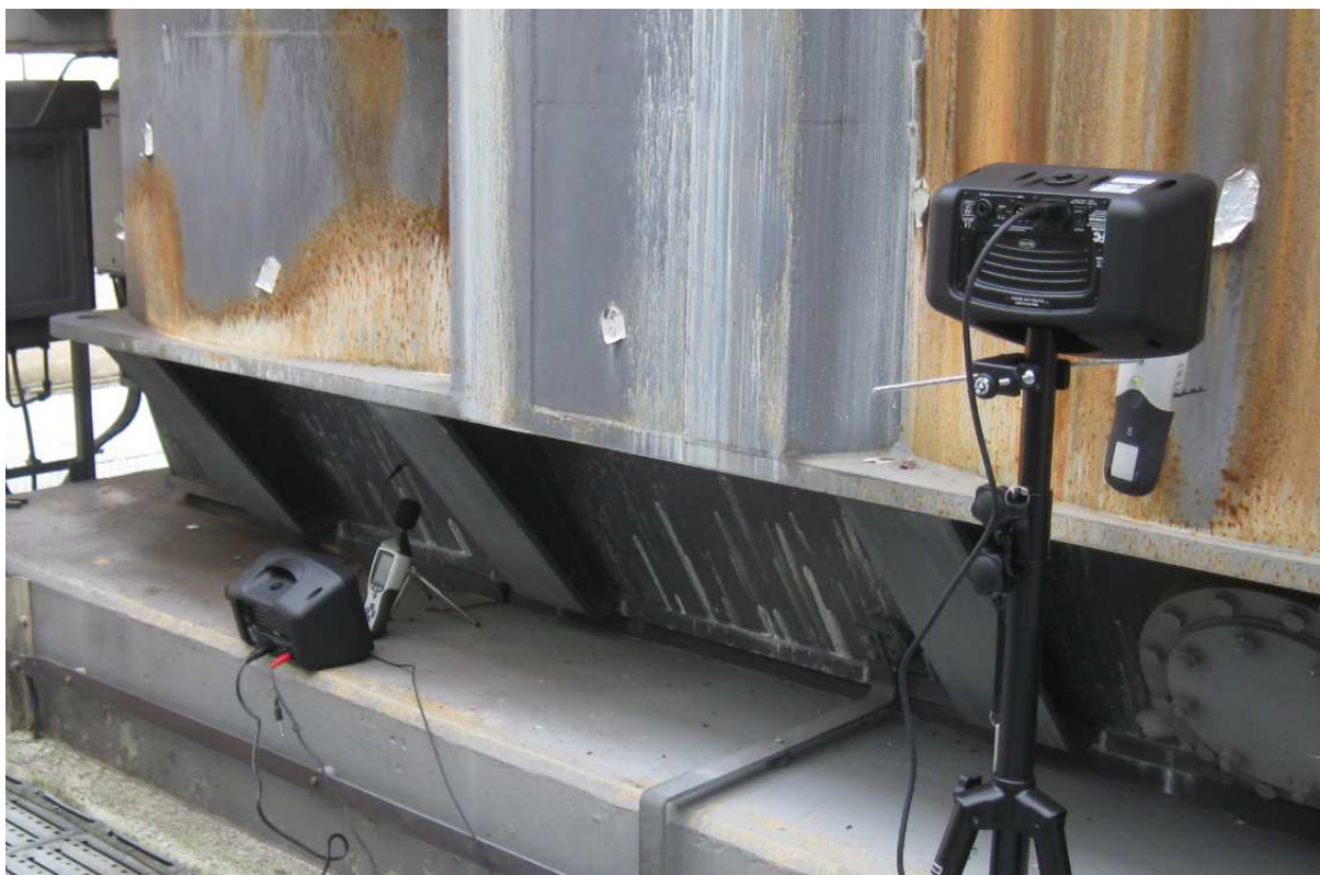
Figure 7 – Loudspeaker positions near parts of transformer
